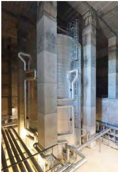
□ The Firstly Built Energy Box in Hamburg
